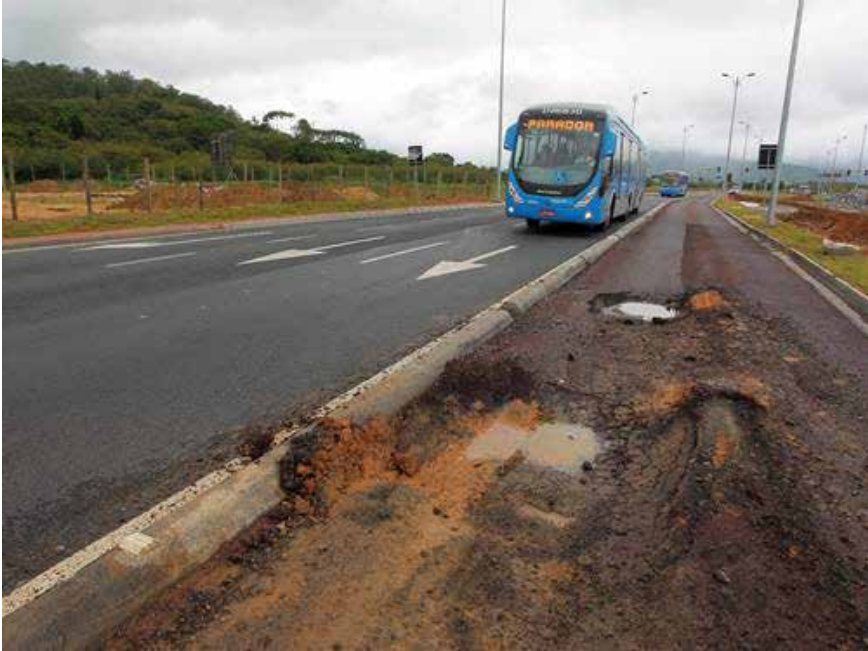
Figure 5 - Picture of Transoeste BRT lane degradations
